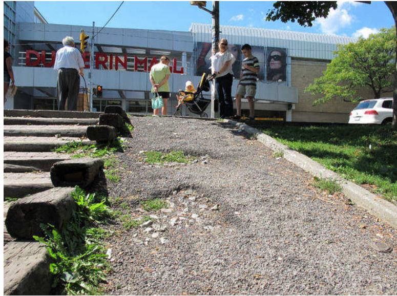
An asphalt ramp leading from a sidewalk on Dufferin St. into Dufferin Grove Park is crumbling and too rough for people who use wheelchairs, motorized scooters or baby strollers.
