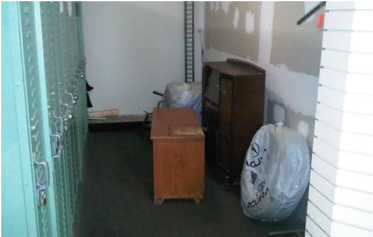
Locker Room at Don Valley Golf Course – lockers are old and need replacements, drywall needs further repair, requires paint, and is being used as storage for items that should not be there including tires
