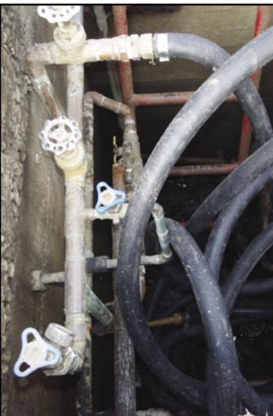
Existing valve pit
