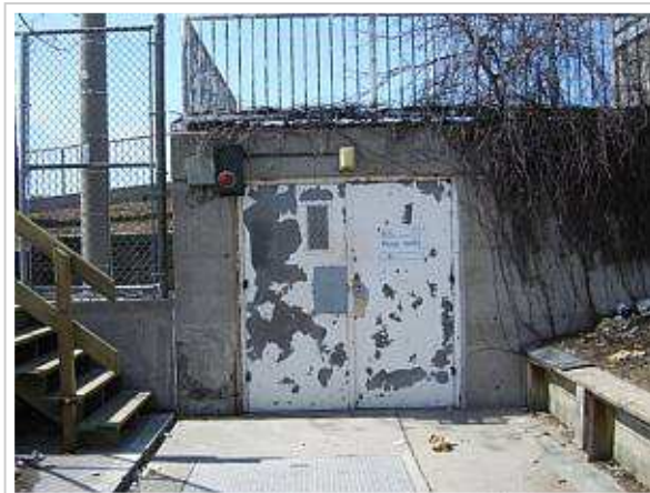
compressor room doors
